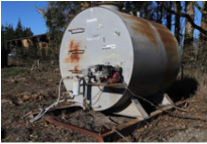
Diesel Tank 5000 Litre
