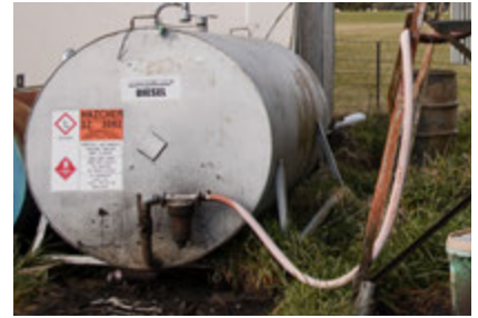
2500L Onground Diesel Tank
