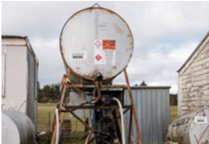
2000L Overhead Fuel Tank. (Electric pump)
